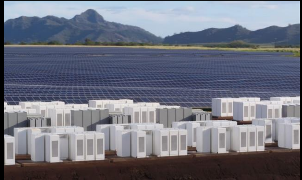
Tesla battery project in Hawaii
