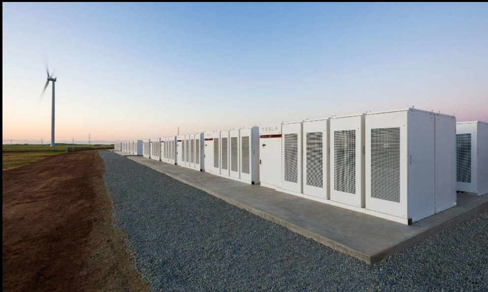
Tesla battery project in Australia
