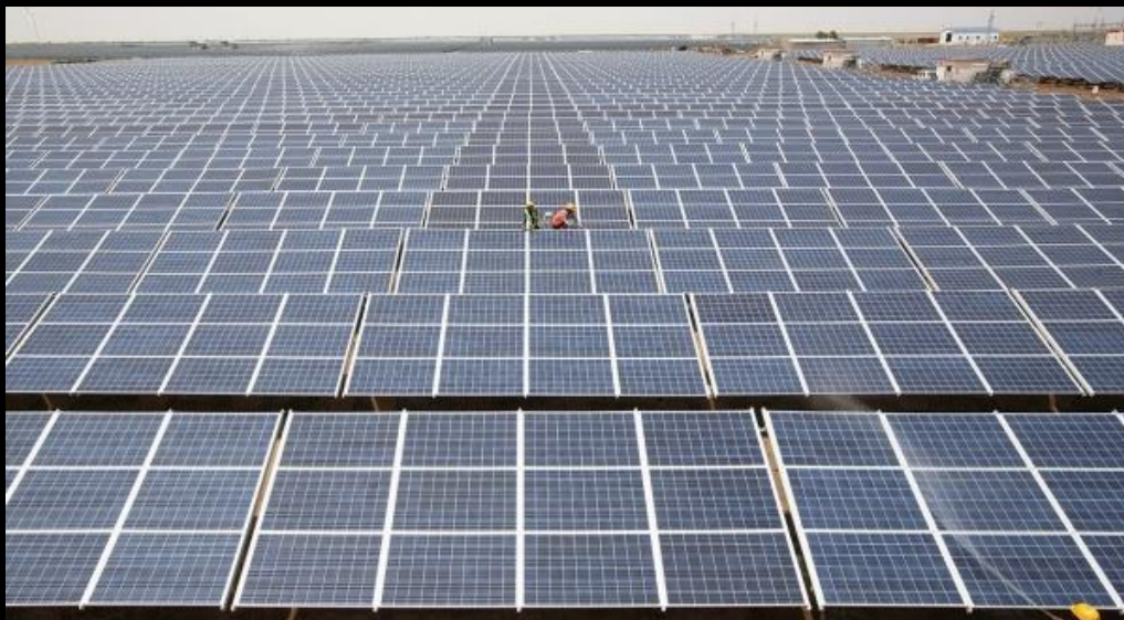
Gujarat solar park, Charanka village, India
